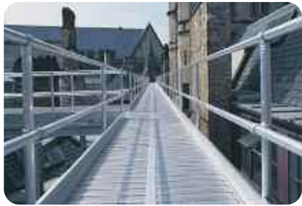
Lightweight Double-Width Spandeck Walkway over roof of old building provides safe access to essential services.
