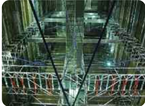
Quick-Erect Boiler Scaffold System at Manjung, Malaysia. View looking from the bottom of the hopper showing the outer support trusses and main tower structure. The boiler scaffold for this 660MW unit was commissioned in 2007.
