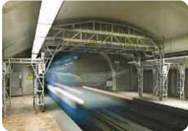
Special Rolling Bridge for Metro Station roof maintenance.
