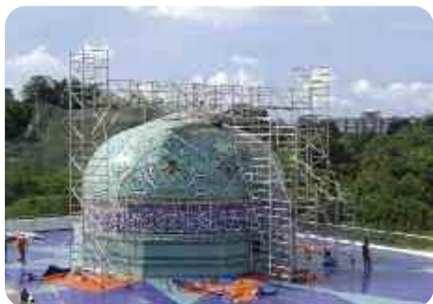
Pool Bridge Scaffold and Cantilever Towers at the mosque in the Kuala Lumpur Federal Government Building, Malaysia.
