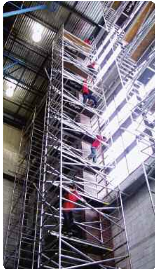
High Towers provide floor-to-ceiling access in large buildings.
