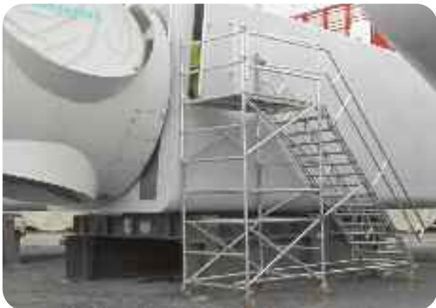
Access Steps for a Siemens Wind Turbine Nacelle (Belfast, Ireland).
